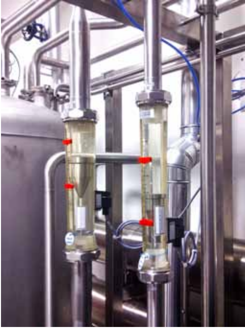
Monitoring of the flow of concentrate and recirculation of a reverse osmosis water treatment plant
