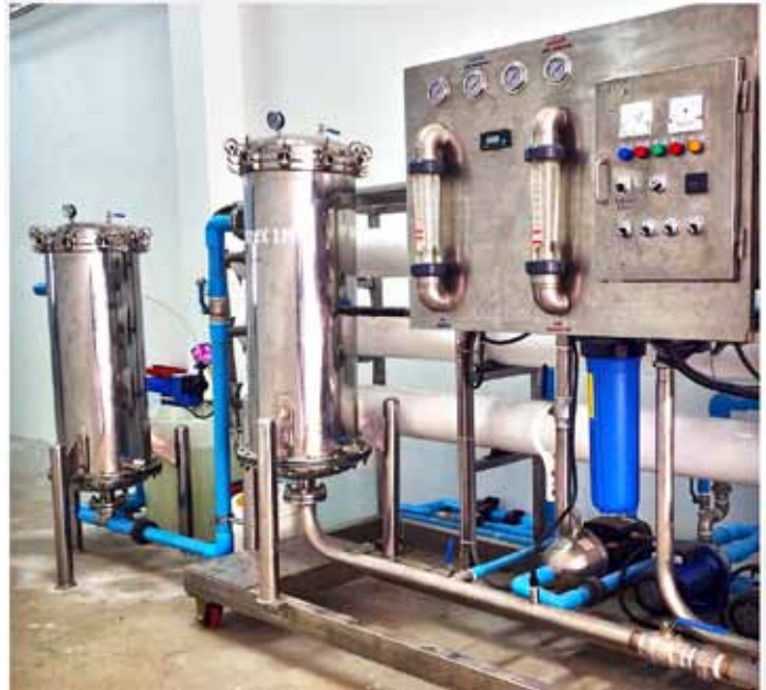
Reverse Osmosis System
