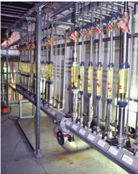
Cooling water distribution system in a glass melting factory
